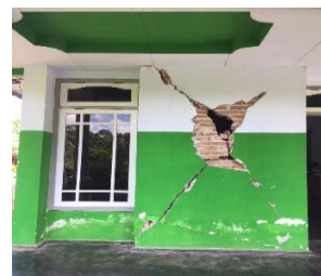
Figure 1. The effect of Earthquake in Malang, 10 April 2021
